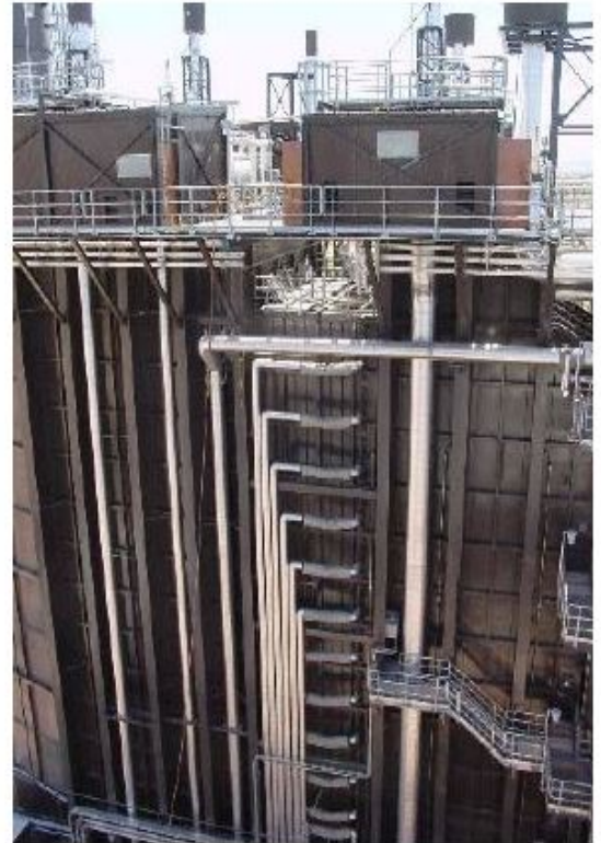
Figure 1: Exterior of an exhaust duct showing the Ammonia Injection Grid
